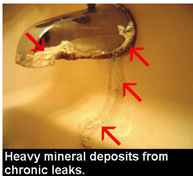
Droplets from a leaking faucet control.
