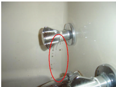
Droplets from a leaking faucet control.
