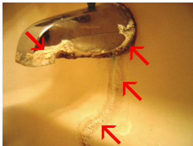
Heavy mineral deposits from chronic leaks.
