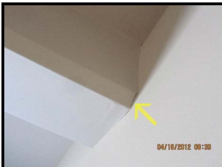
Wall / ceiling cracking
