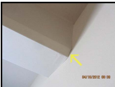
Wall / ceiling cracking
