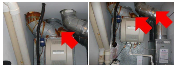
RUST NOTED ON FURNACE FLUE PIPE
