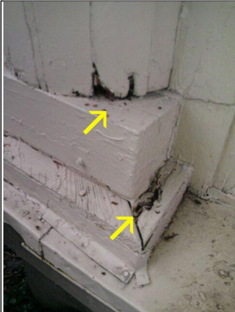
Wood rot present
