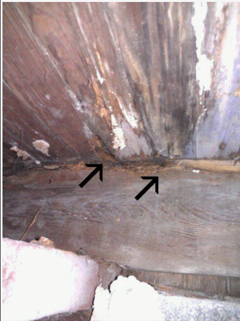
Joists rotted in some locations
