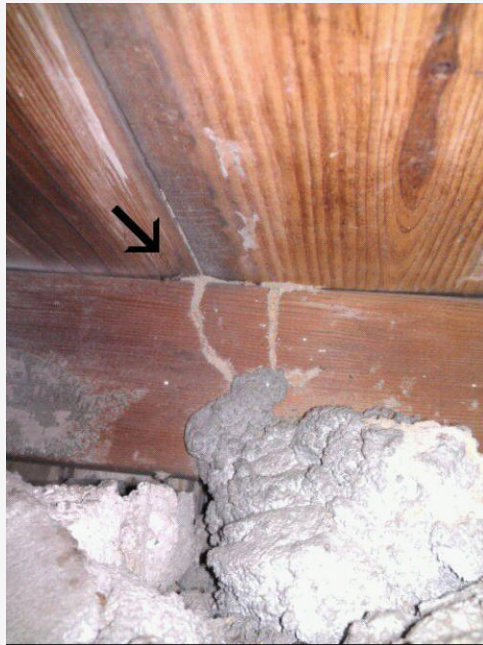
Termite shelter tubes
