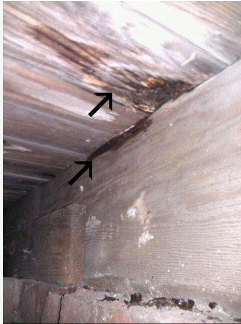
Water damage /rot
