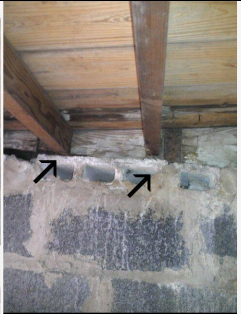
substandard floor framing below kitchen
