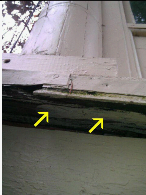
Rot present under capping
