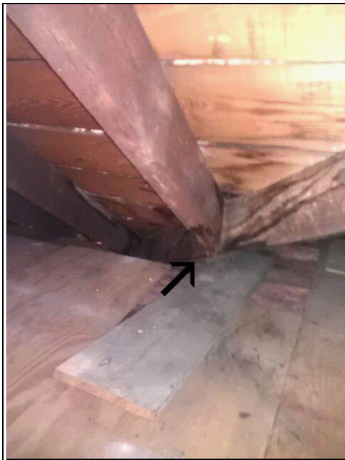
Evidence of previous leakage.
