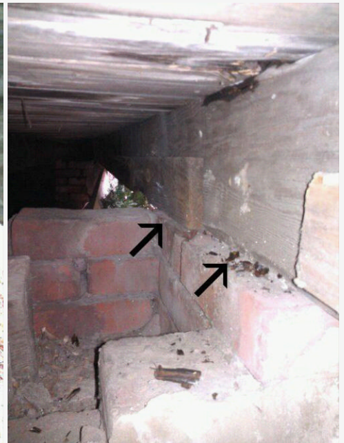
Improperly supported joist
