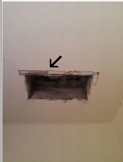
Knob and tube wiring at fuse box in closet
