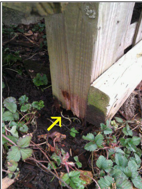
Base of post is rotted.
