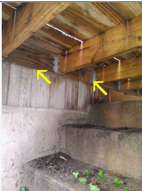
Deck improperly supported
