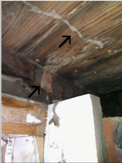
Termite shelter tubes / damaged wood
