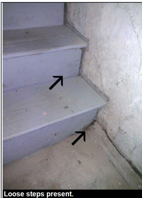
Loose steps present.
