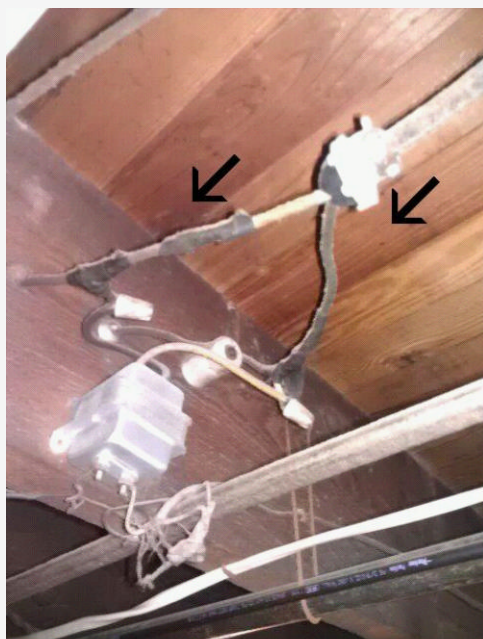
Knob and tube wiring / improper splices
