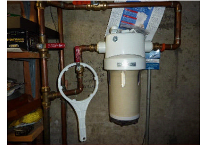
Whole house filter
