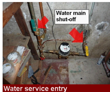
Water service entry
