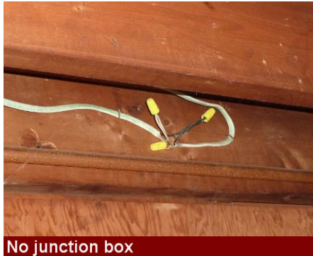
No junction box
