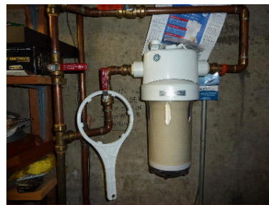
Whole house filter
