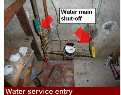
Water service entry
