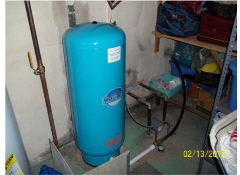
Tank & pump control switch
