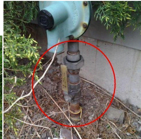
Gas service shutoff valve
