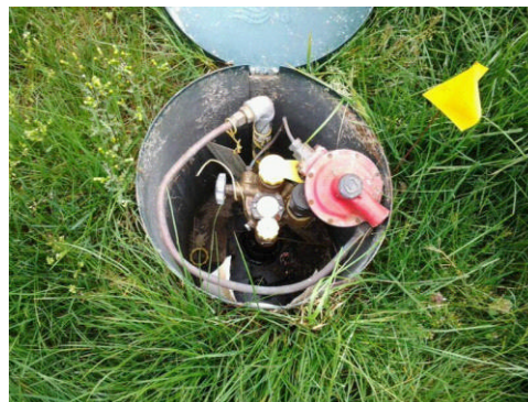
Buried propane tank
