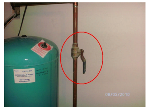
Water main shutoff valve
