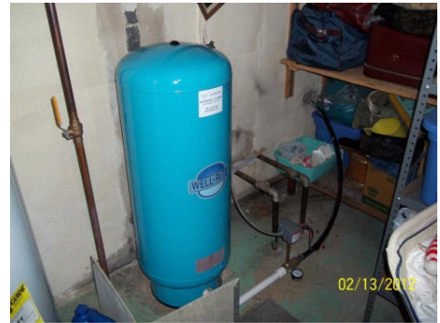
Tank & pump control switch
