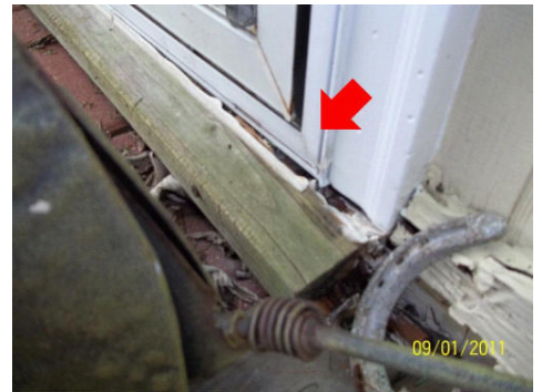
Door still needs repaired.
