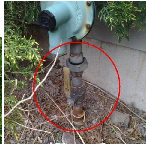
Gas service shutoff valve
