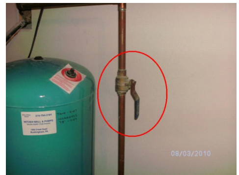
Water main shutoff valve
