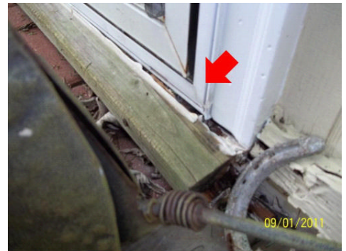
Door still needs repaired.
