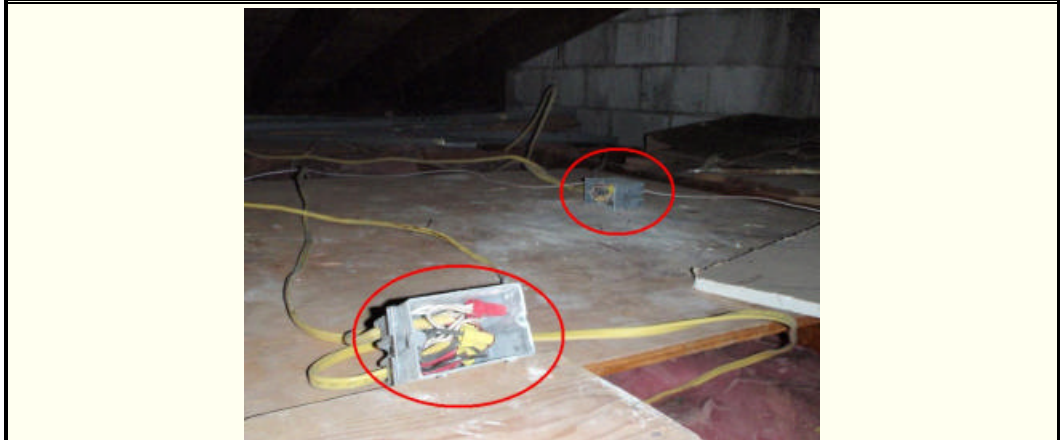
Open junction boxes in the attic.
