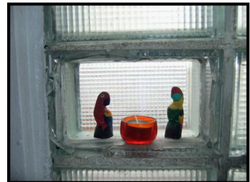
BROKEN/CRACKED GLASS BLOCK
