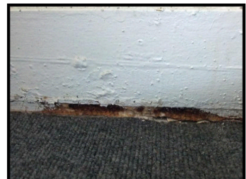
WATER STAINS AT THE RIGHT WALL
